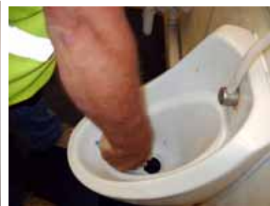
Clean old sealant from urinal to ensure that new fitting seals properly
